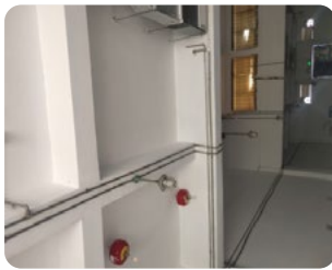
▲ Explosion-proof lights/ explosion-proof lines
